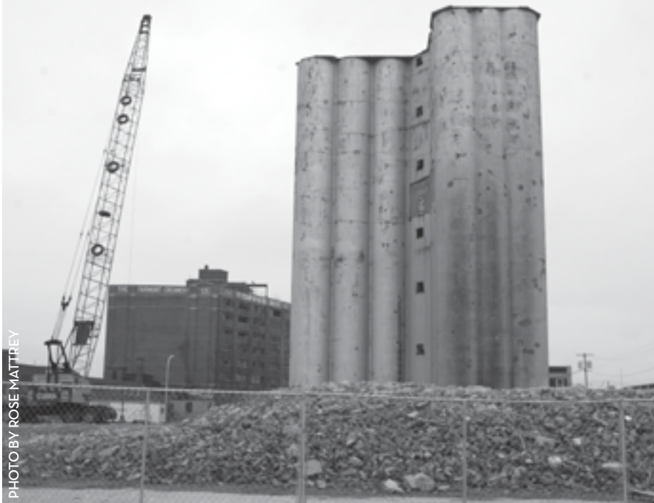
Demolition has begun already on the property the Seneca Nation has acquired for the proposed Buffalo Creek Casino.
